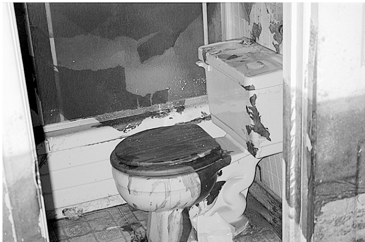
Figure 1.2.1D: The result of sewage back-up through a toilet during a riverine flooding event
